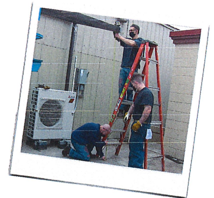
Right: Metal shop orderly Daniel Carter and welding assistant Gerry Hight help lead-welder Nicholas Escriva install an awning over the electrical shop entrance.
